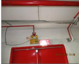
Photo of fire safety equipment Exit sign.JPG
