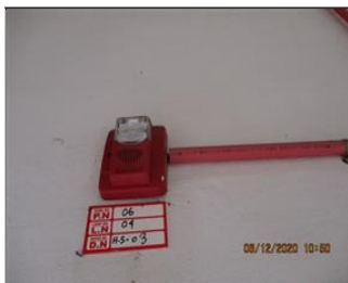
Photo of fire safety equipment Fire alarm.JPG
