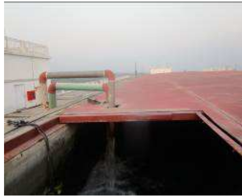
I001) Incoming Water - Surrounding (GPS Location: N 23° 48' 0"; E 89° 13' 0.12")
