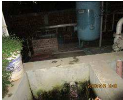
I002) Wastewater After Treatment - Surrounding (GPS Location: N 23° 48' 0"; E 89° 13' 0.12")
