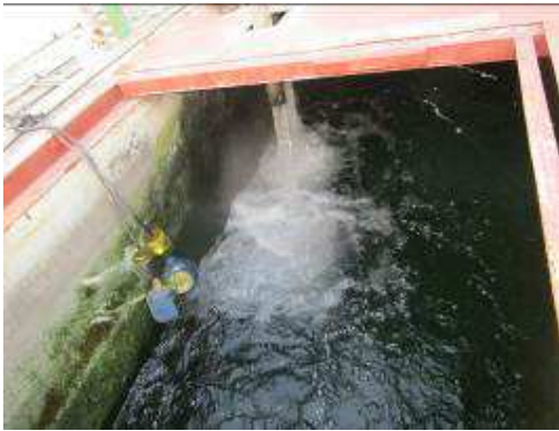
I001) Incoming Water (GPS Location: N 23° 48' 0"; E 89° 13' 0.12")
