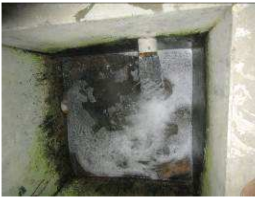
I002) Wastewater After Treatment (GPS Location: N 23° 48' 0"; E 89° 13' 0.12")
